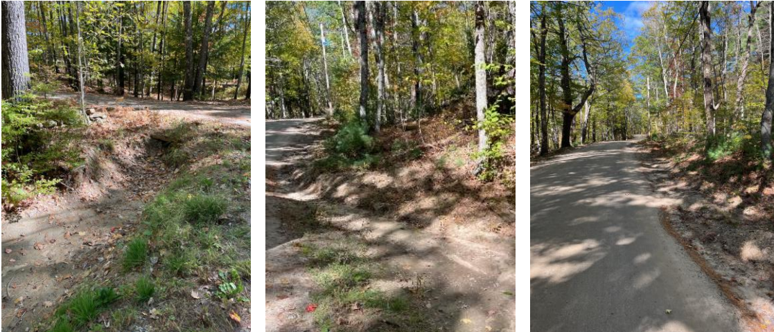
(Left) The culvert inlet has bare soil. (Middle) The end of the gully is a wide, bare soil area. (Right) The gully extends 500 feet up the road.
