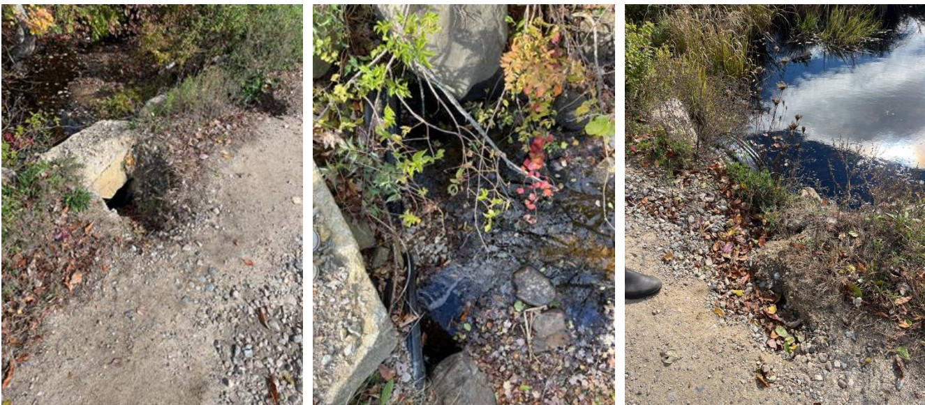
(Left) Severe erosion at the culvert outlet. (Middle) View of twin culverts. (Right) There is minor erosion at the culvert inlet.
