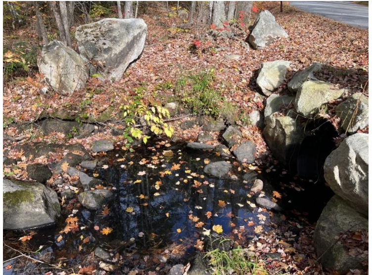
An undersized culvert is causing bank scours at the culvert outlet.
