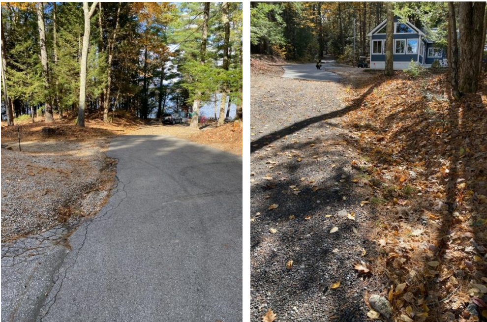
(Left) View of Pine Point Road shoulder facing the lake, (right) View of the road shoulder gully facing up hill, away from the lake.
