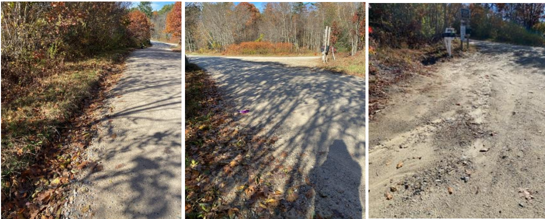
(Right) Southern road shoulder of Old Richie Road facing downhill towards its intersection with Northwood Lake Road (middle and right).
