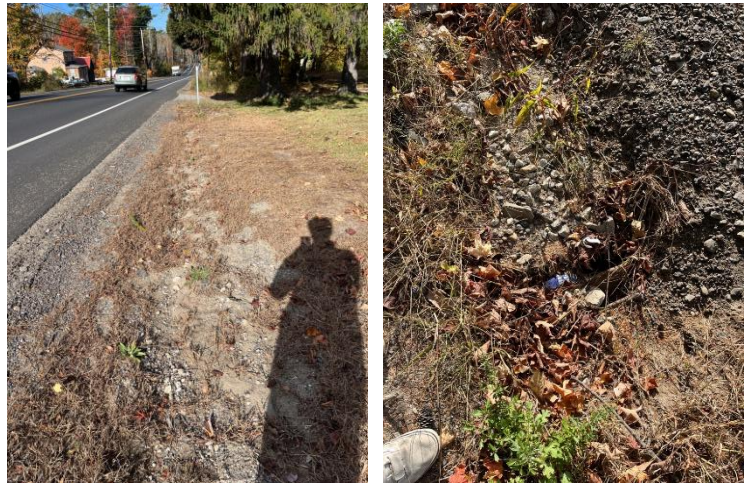
(Left) Road shoulder erosion leading to a catch basin. (Right) The catch basin is buried in gravel.
