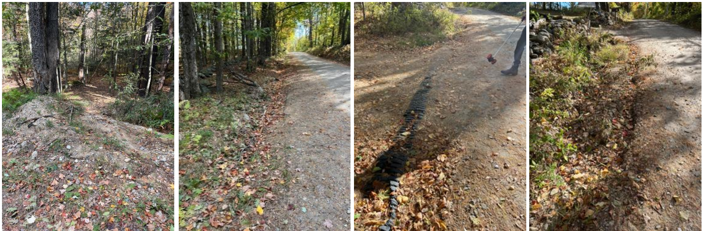
(1) The turnout on Range Road has accumulated sediment at its end. (2) The road shoulder ditch is eroding. (3) An under-driveway culvert is exposed. (4) The road surface of Range Road is eroding.
