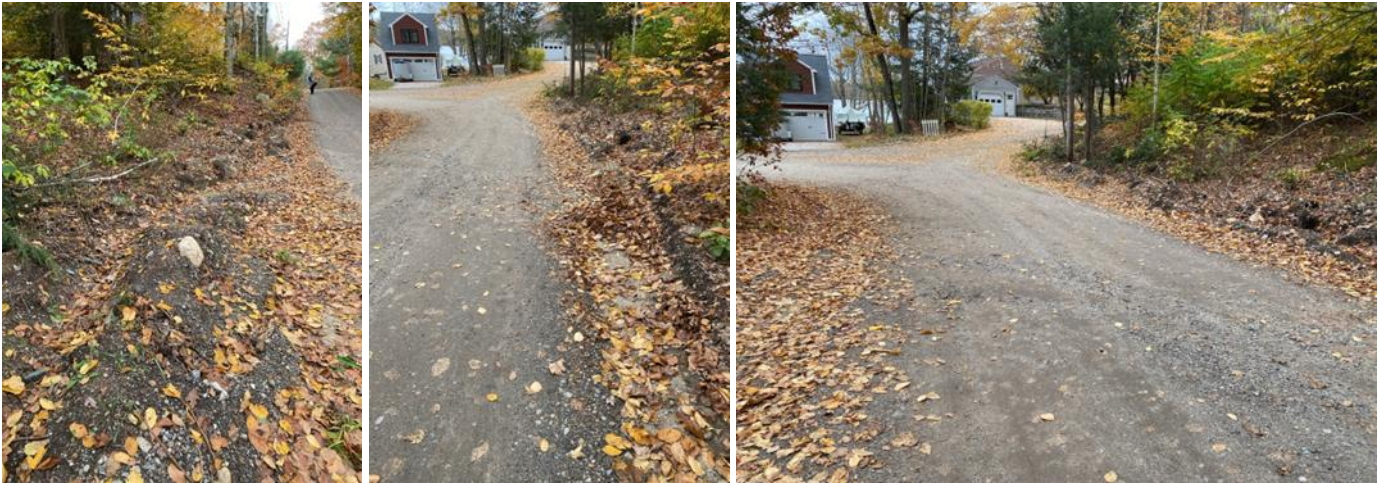
(Left) Southern road shoulder gully looking uphill. (Middle) Southern road shoulder gully looking downhill. (Right) Flow path of the road shoulder flow crossing Birch Street to the intersection with Shore Drive.
