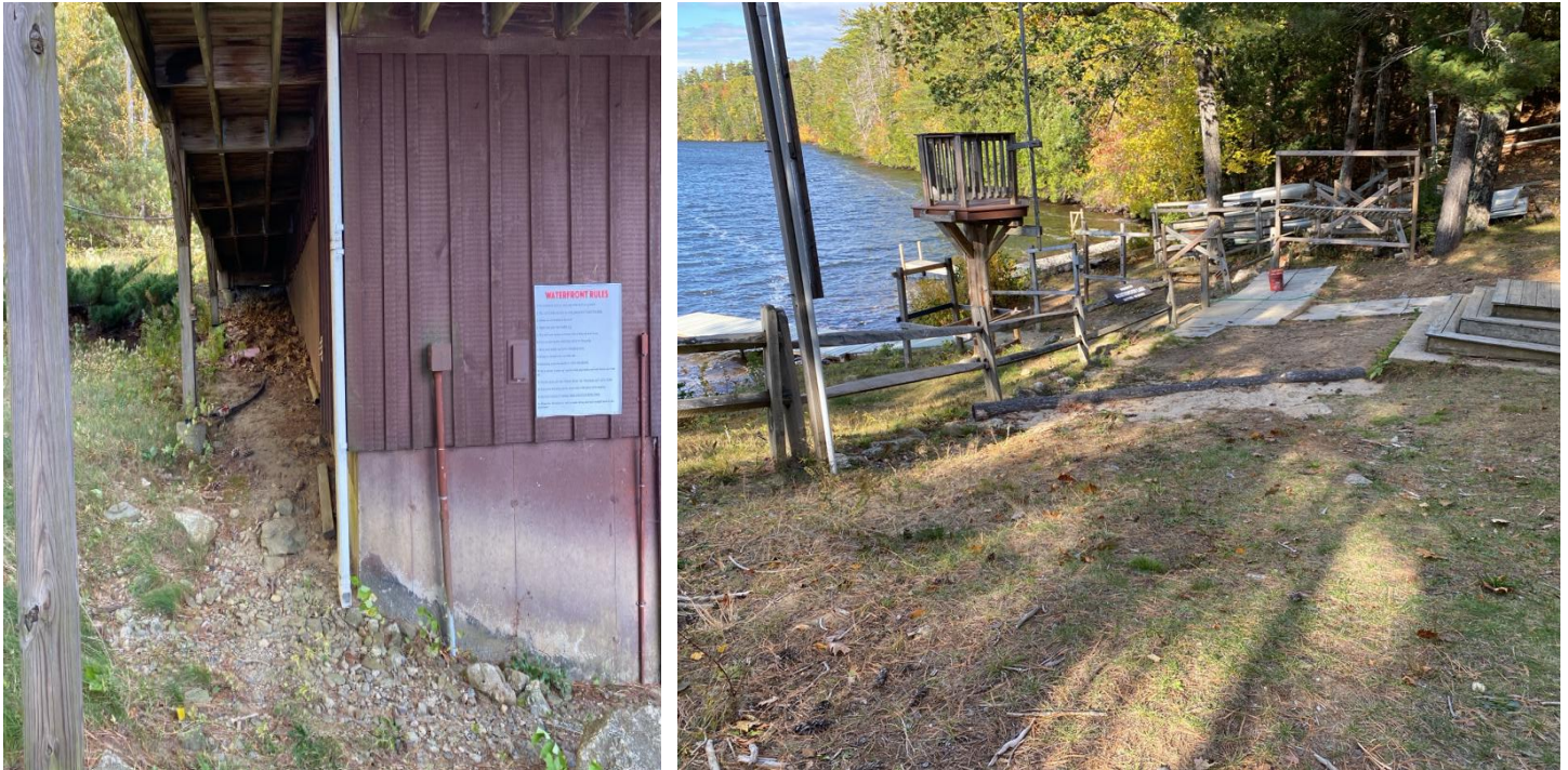
(Left) the evidence of erosion from roof runoff prior to gutter installation along with the white gutter downspout. (Right) the water access area sloping to the lake with fencing to define access points.
