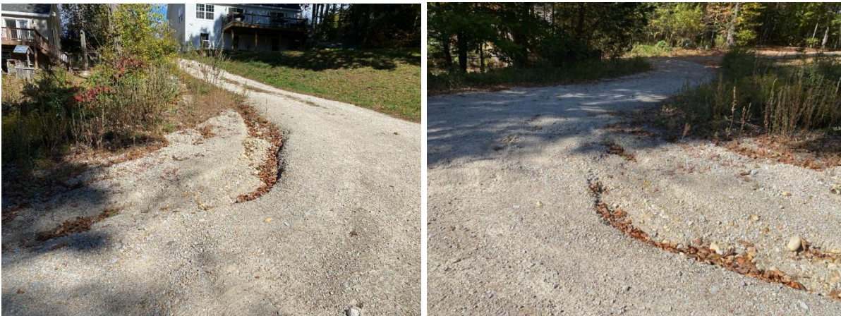
Erosion gully at the base of the driveway turning onto Maple Avenue.
