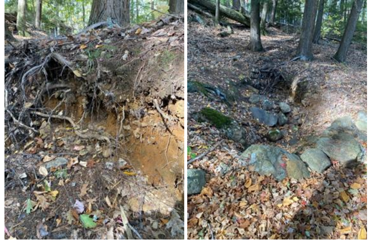
(Left) The upgradient side of the culvert showing the large, eroded basin. (Right) View of the eroded soils and exposed tree roots on the upstream side of the culvert.
