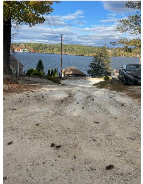
Road surface erosion on Lynn Lane leading to Northwood Lake.
