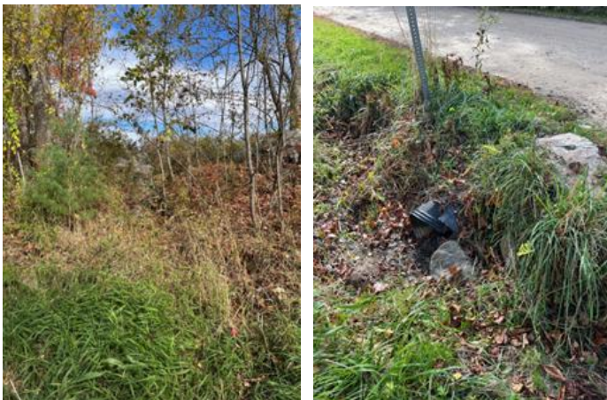
(Left) Trail of rip rap leading from an agricultural property to the road shoulder ditch, obscured by vegetation in the photo. (Right) Slightly crushed culvert outlet at the site.
