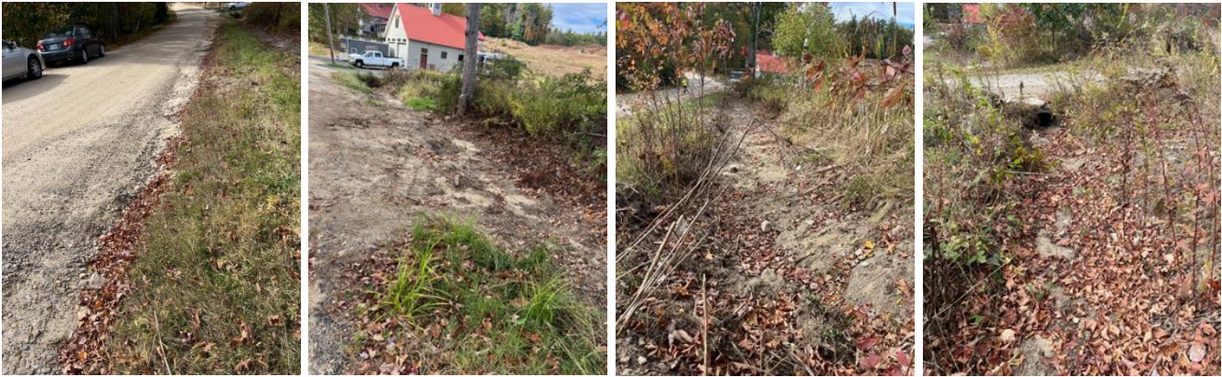
(Photos 1-3) Road surface erosion in addition to road shoulder ditch erosion. (Bottom Left) Stormwater is eroding the road surface. (Photo 4) Stormwater enters water resources through a culvert.
