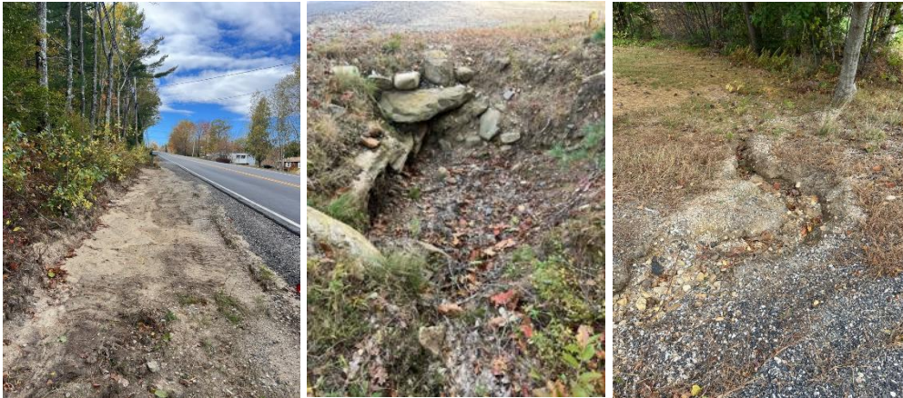
(Left) The road shoulder is composed of loose, bare sand. (Middle) The culvert inlet also shows signs of erosion. (Right) The gully created by the outflow.
