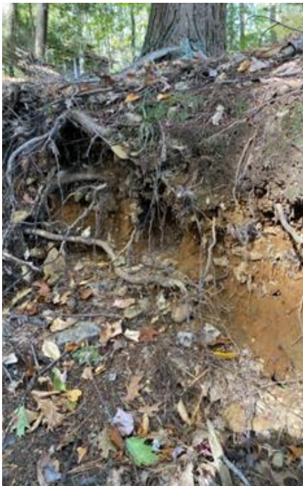
The upgradient side of the culvert showing the large, eroded basin.
