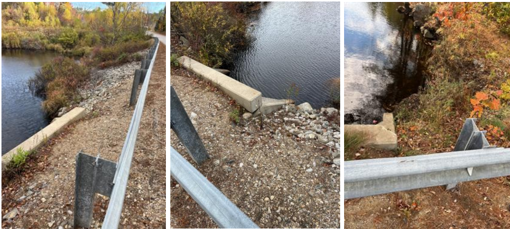
(Left) The bare road shoulder above the culvert outlet site, (middle & right) stormwater has eroded the shoreline, providing paths for stormwater to directly enter Tucker Brook.
