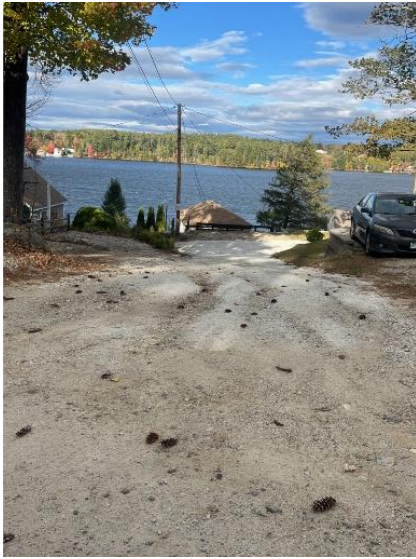
Road surface erosion on Lynn Lane leading to Northwood Lake.
