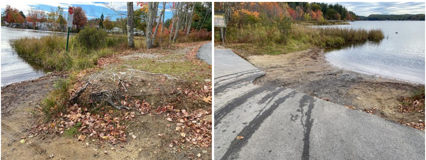
(Left) Exposed roots and a steep drop off of the shoreline to the water's edge indicating erosion, (right) the end of the paved boat ramp where it meets the water.
