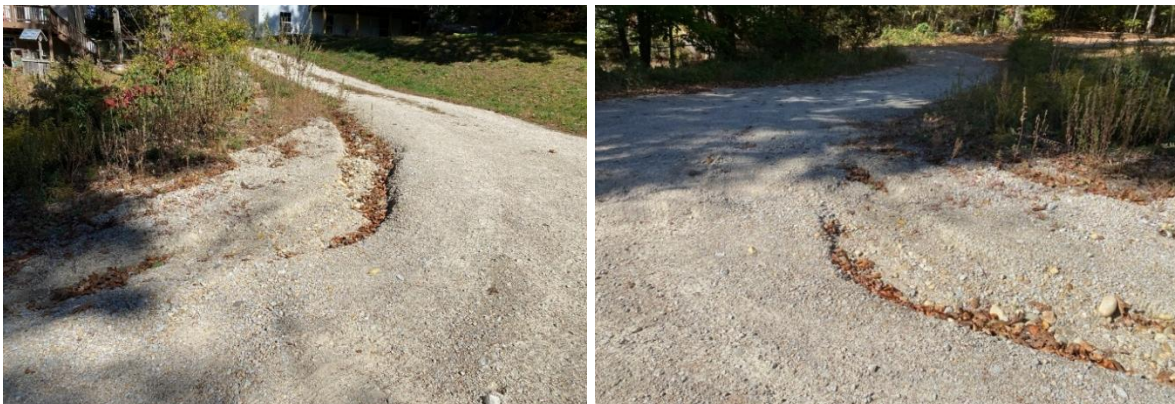
Erosion gully at the base of the driveway turning onto Maple Avenue.
