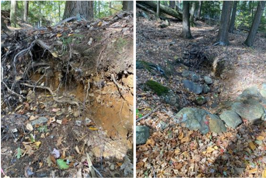
(Left) The upgradient side of the culvert showing the large, eroded basin. (Right) View of the eroded soils and exposed tree roots on the upstream side of the culvert.
