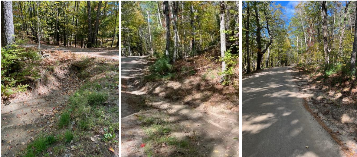
(Left) The culvert inlet has bare soil. (Middle) The end of the gully is a wide, bare soil area. (Right) The gully extends 500 feet up the road.
