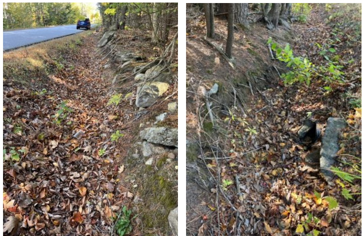
(Left) Road shoulder erosion leading to a catch basin. (Right) The catch basin is nearly completely buried in gravel.
