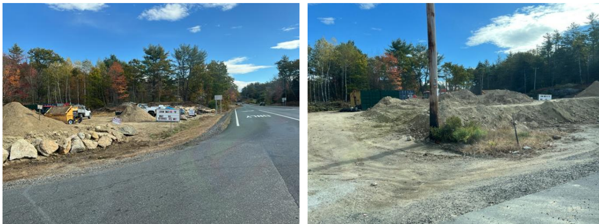
Bare soil and sediment piles at the construction site on Route 4.
